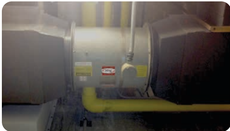
Series 28 Fiberglass Direct Drive Duct Fan in Caustic Soda Room at a Water Treatment Plant
