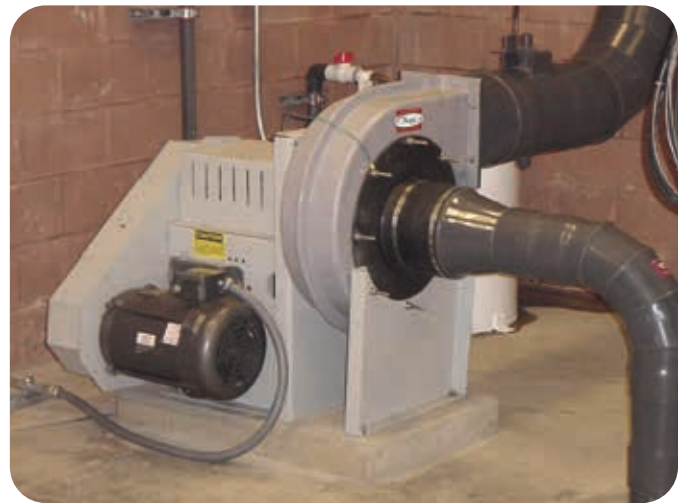
Series 43 Fiberglass Radial Blower at a Pump Station
