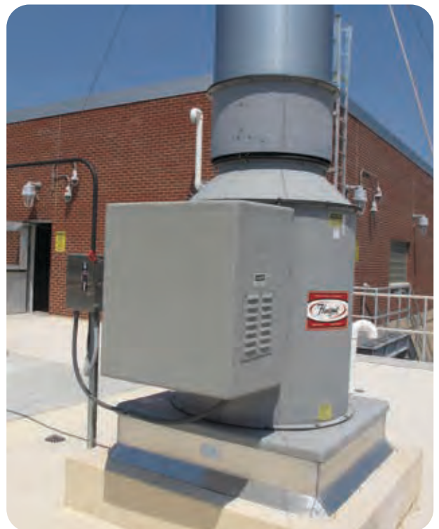
Series 40 Fiberglass In-Line Centrifugal Fan at a wastewater treatment plant.
